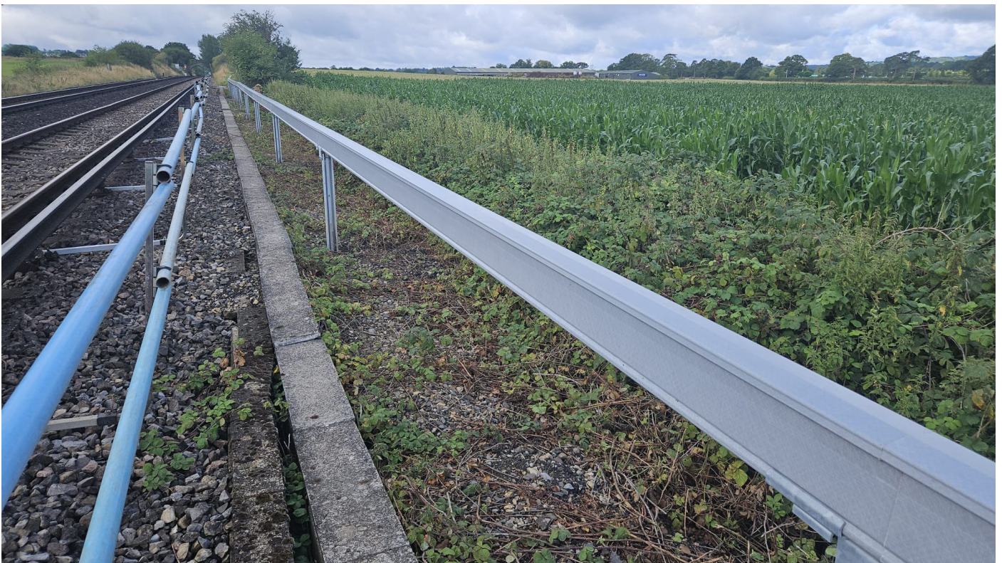
ARCOSYSTEM® cable troughing installed trackside via ground-mounted posts
