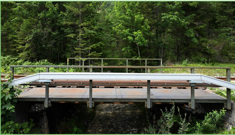
ARCOSYSTEM® safely fastened to the side of a bridge in order to maintain the cable run
