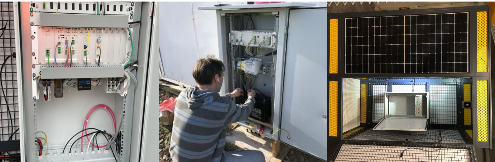
Installation of external cabinet, DMP Rack located in SolarXBox
