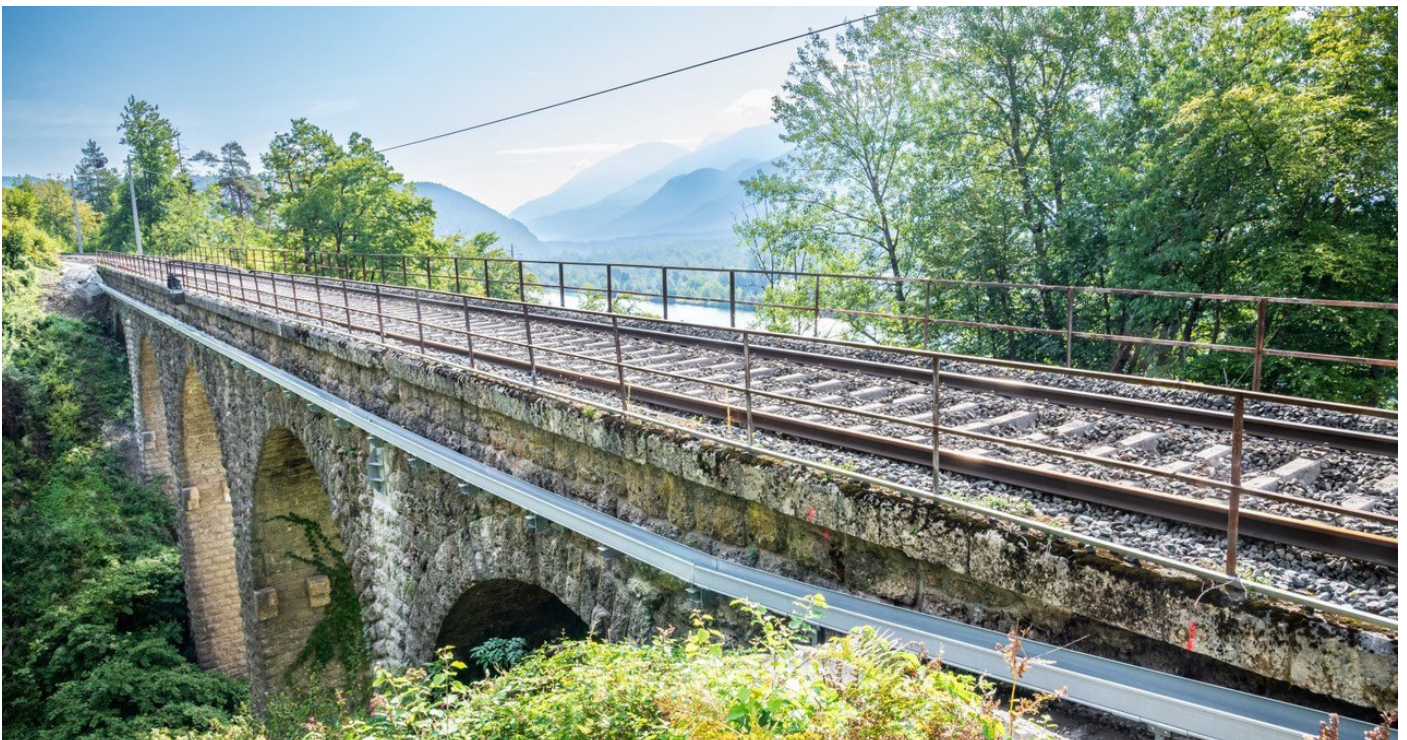
ARCOSYSTEM® troughing attached to the side of a stone bridge near Klagenfurt, Austria
