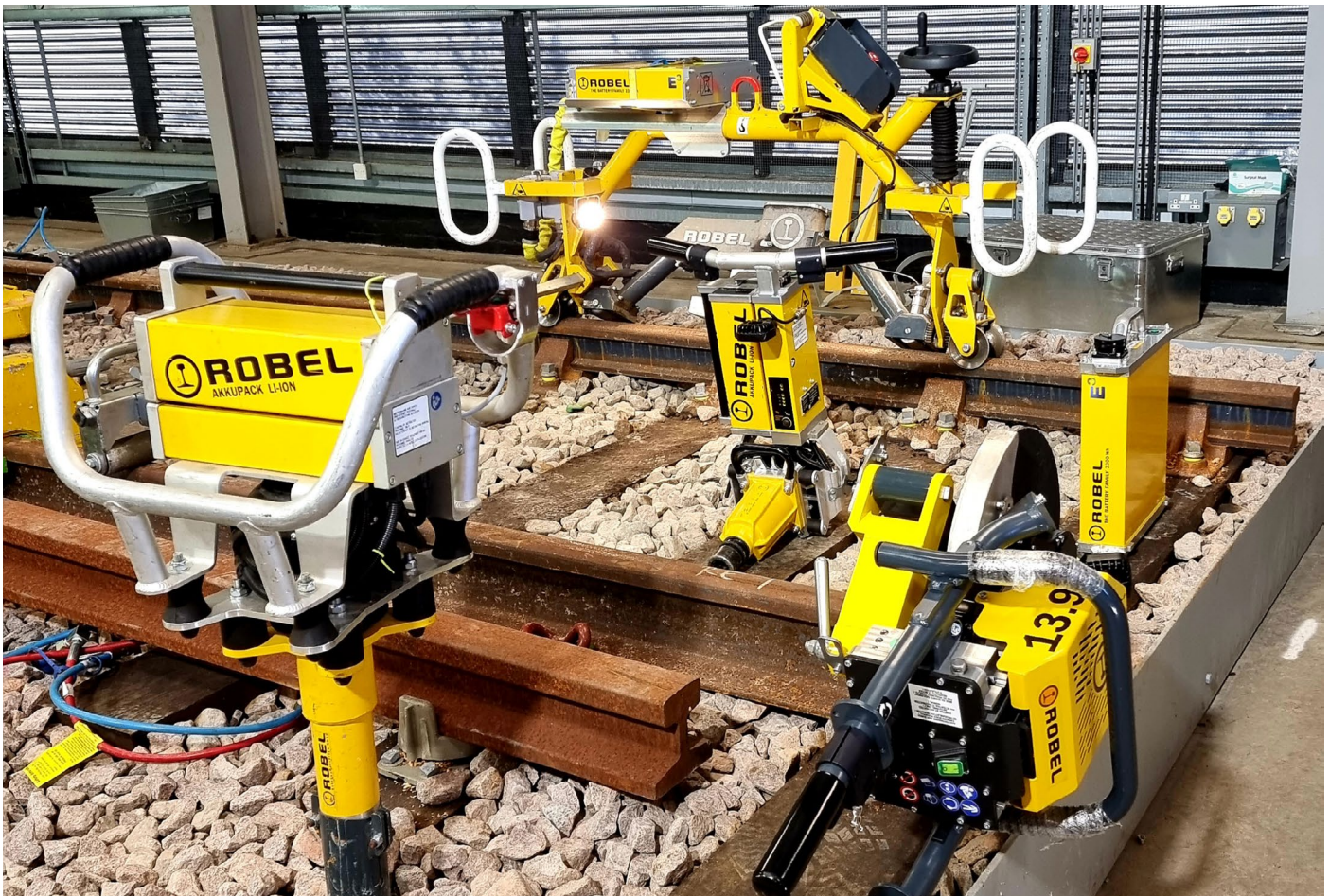
The battery-powered E 3 construction site – from left: ROTAMP 62.20L, ROGRIND 13.49, ROMPACT 30.20, ROCURT 13.90 © Robel
