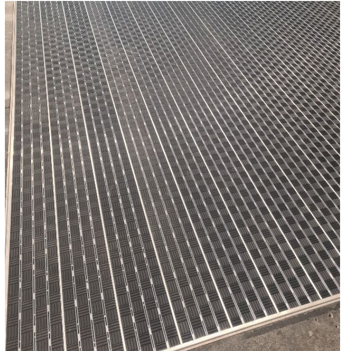
Installation of EMS Multi-track Natural (section 12) Entrance Matting installation at Romford Station
