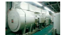
Flywheel-type train line power storage equipment
