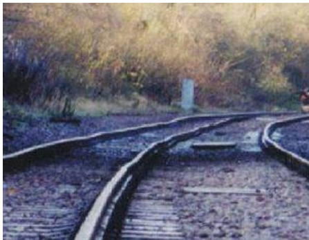
Figure 2. Misaligned Track Section Due to Subgrade Pumping
