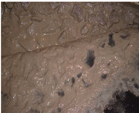
Figure 9. Underside of Geocomposite after 70 Million Gross Tons of Loading
