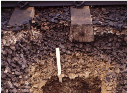
Figure 1. Ballast Contaminated with Subgrade Fines
