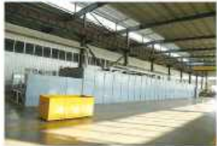
Veneer drying line
