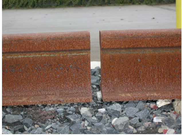
Figure 8: Rail ends not cleaned - Incorrect
