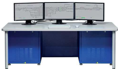
Station operator work terminal ARM DSP
