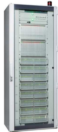
Main interlocking control unit UKTs
