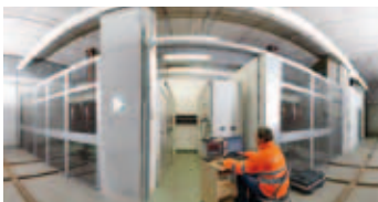
METRO BILBAO INGEBER energy recovery system: 5 units.
