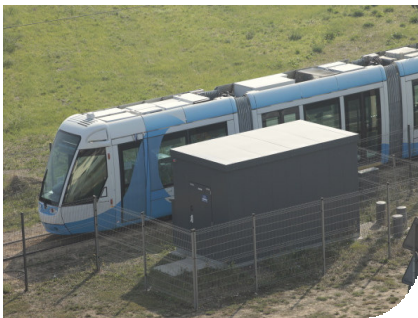
A HESOP substation in testing on a La Rochelle experimental track in September 2009.
