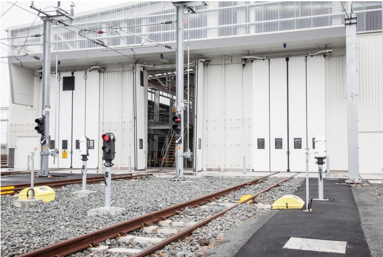
Fig 5: Zonegreen's Intelligent powered derailleurs and signalling systems control depot train movements in a safe and efficient manner
