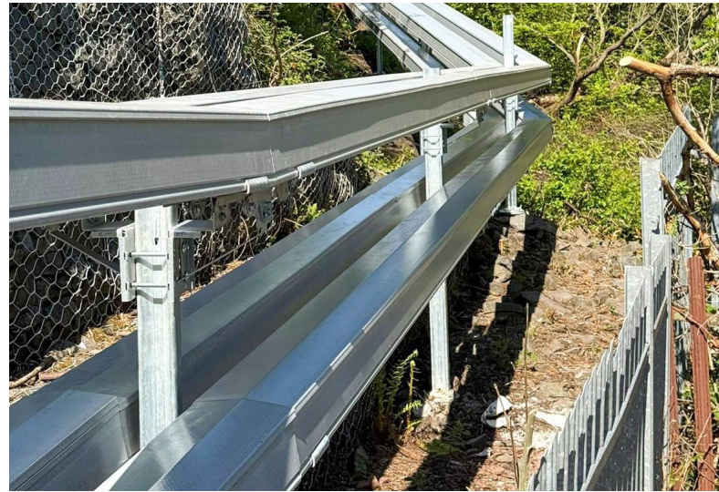
ARCOSYSTEM® installed using the Rapid Route technique with ground-screwed Anchor Screws to ensure solid fitting along a steep trackside route near Glasgow
