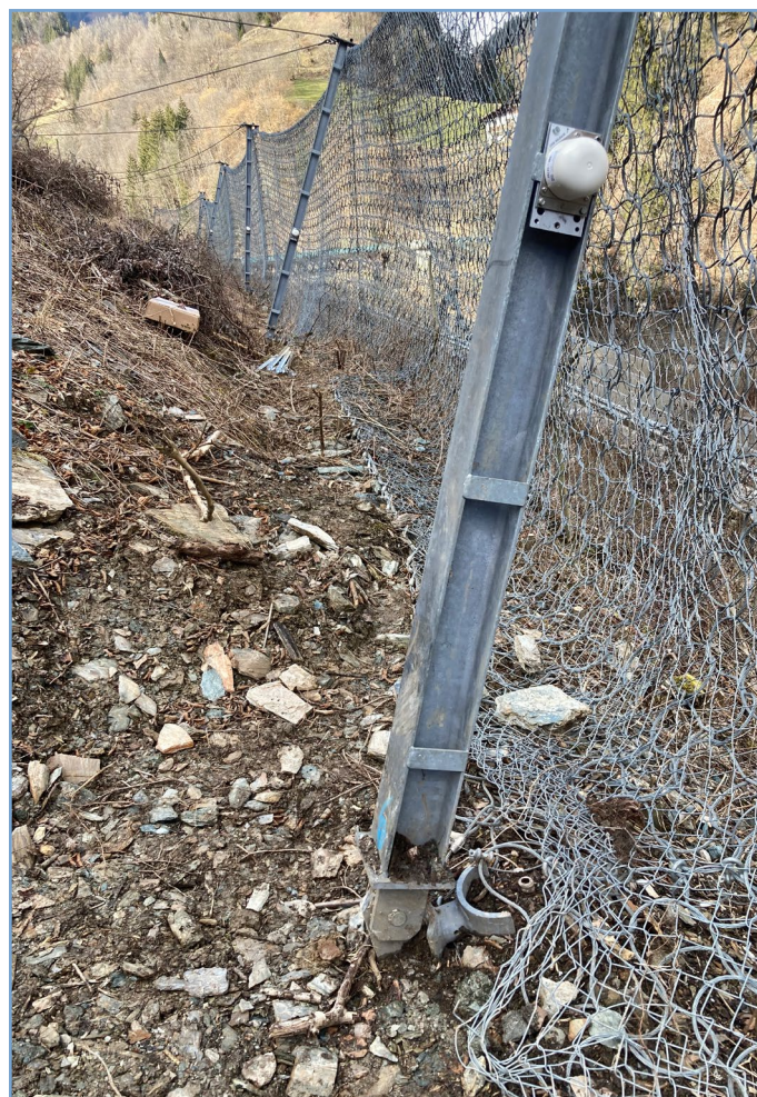
Figure 4: NanoMacro tilt sensor fixed to fence protecting an Austrian railway
