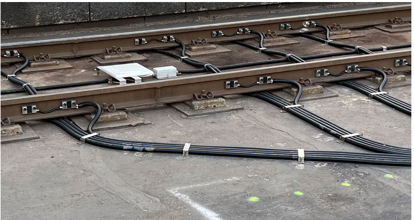
Dynamic Weighing System: measures axle loads, wheel loads, total tram weight and balance dynamically as trams pass at regular speeds
