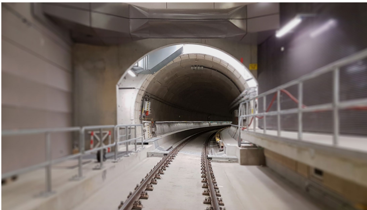
The metro line (52) runs from Amsterdam-Noord under the centre of Amsterdam to Zuid station. Thanks to the application of Amorim Rail Pads, the vibrations and noise at source are reduced, avoiding disturbance to the residents of Amsterdam as much as possible
