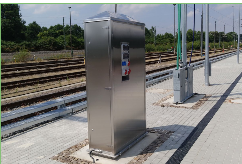
Stainless Steel Cabinet in Chemnitz, Germany (DB)
