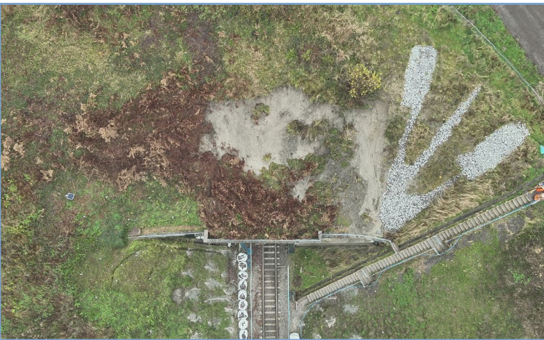
Figure 2: Wireless monitoring is routinely used by Network Rail for early warning of slope failures such as this one at Crewkerne, Somerset
