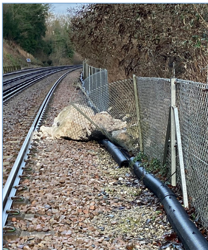
Figure 1: Fences and barriers do not always prevent falling material reaching the track
