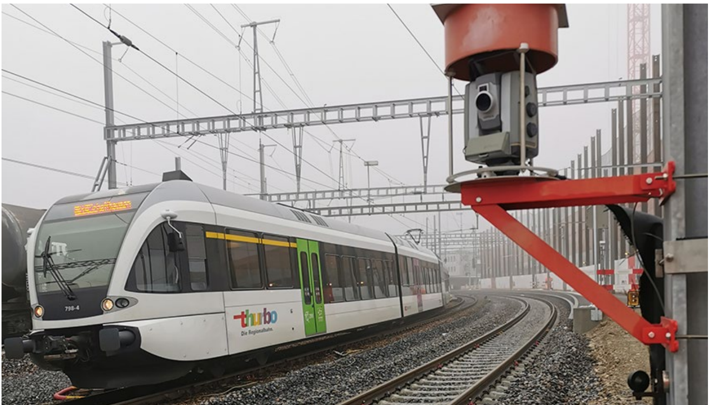
Trimble S7 total station with the construction site for the renovation of the railroad station in Wil (Canton of St. Gallen, Switzerland) in the background
