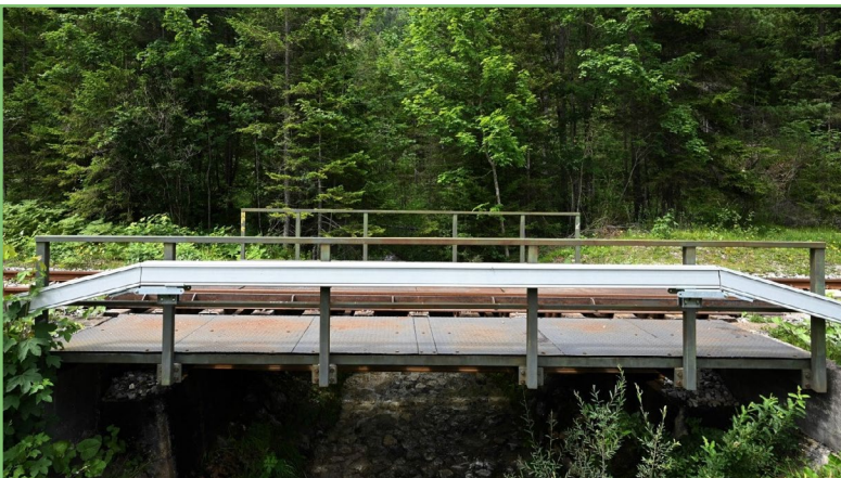
ARCOSYSTEM® safely fastened to the side of a bridge in order to maintain the cable run
