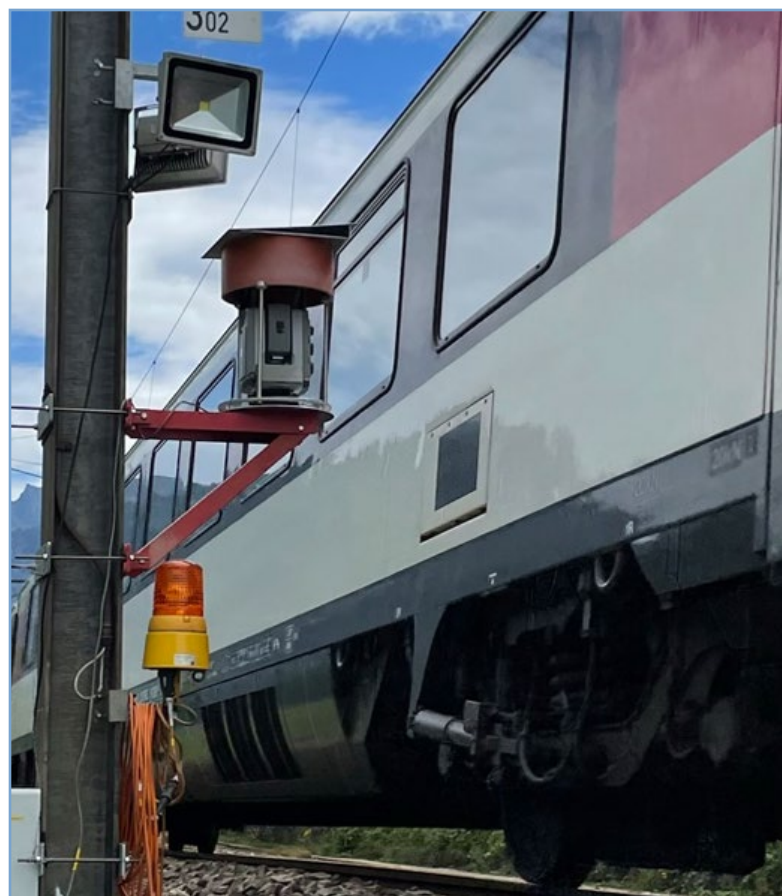
Monitoring of the left track over a length of 450m with five total stations
