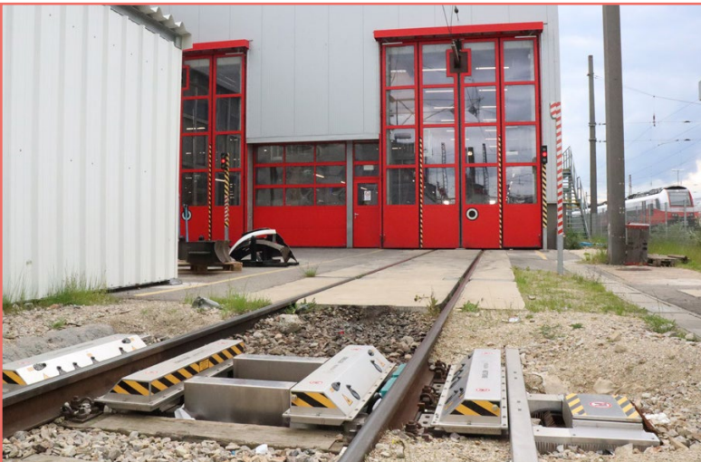
By the time the vehicle comes to a standstill in the hall, all wheelset data is already automatically saved in the system
