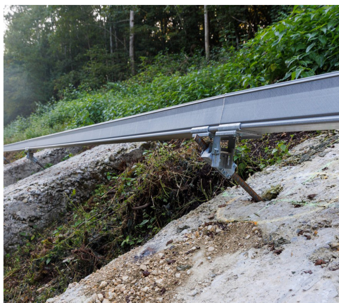
The run of troughing attached to the rock face with the aid of ClickFit brackets
