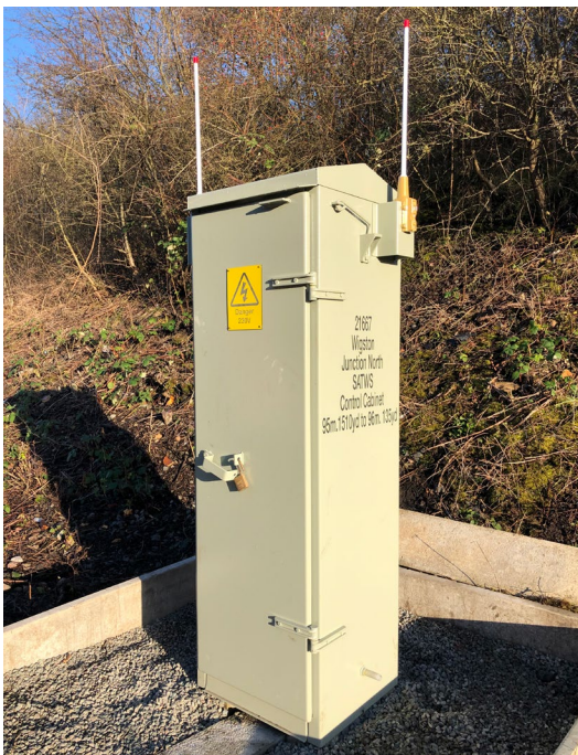
The trackside cabinet houses the transmitters, axle counters and control unit of the permanently installed warning system
