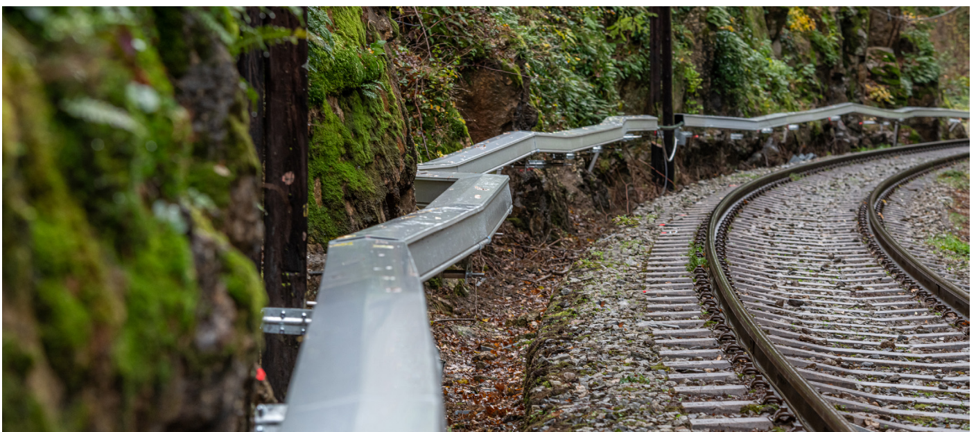
ARCO troughing clamped to lineside rock face in Grein, Austria
