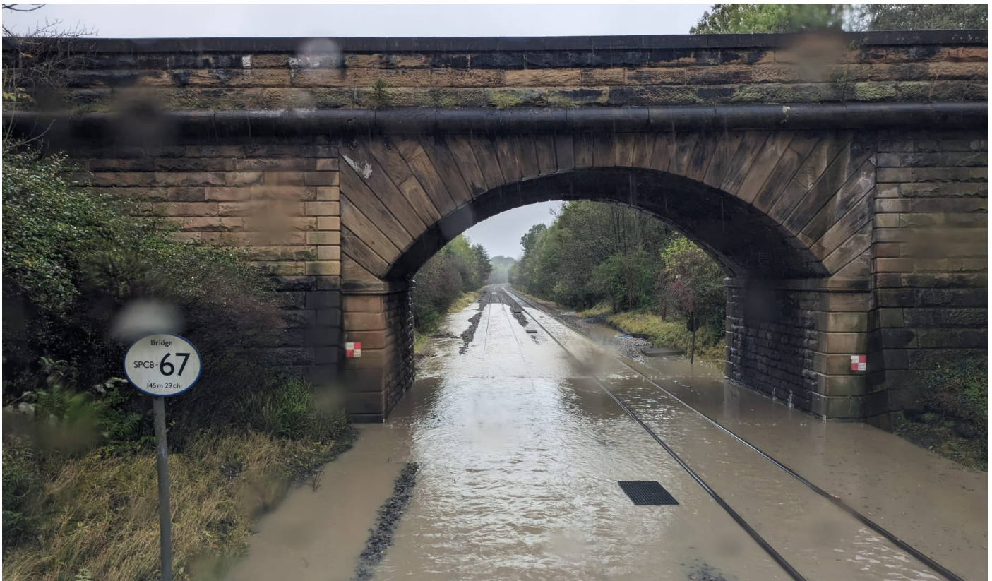
Flooding at Clay Cross © Network Rail
