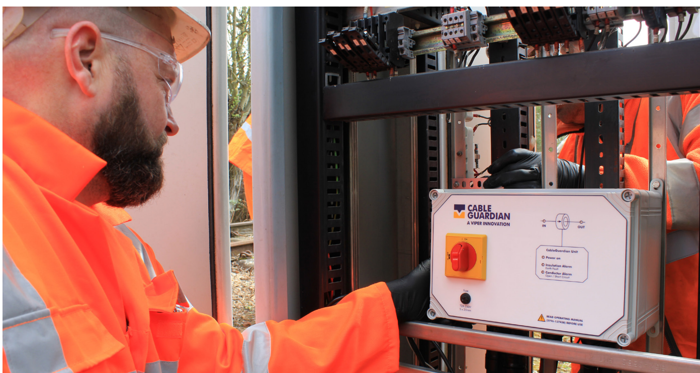
Network Rail rolls out CableGuardian technology across multiple regions
