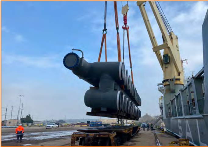
Each slug catcher measured approximately 26 x 4 x 4 m and weighed 196.7 MT
