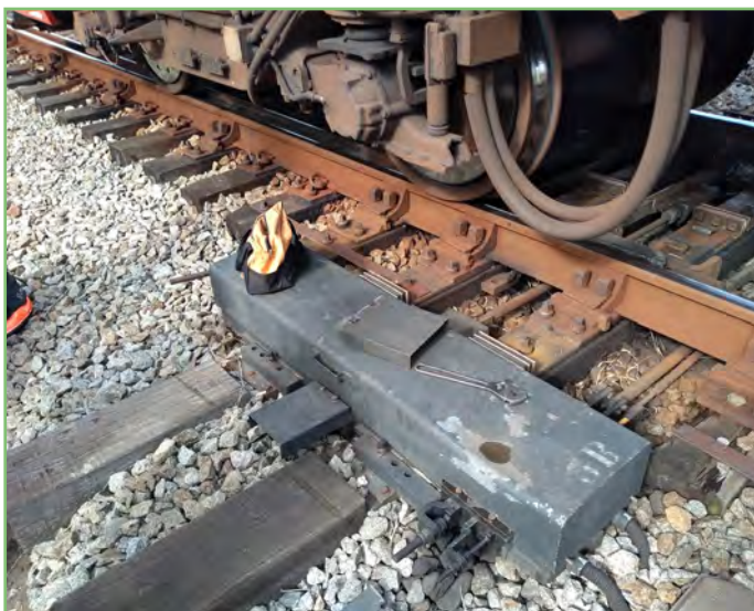
Signalling cable fixation with box Brazil
