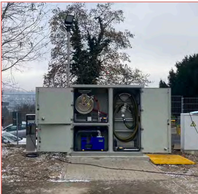
Stand-alone supply & disposal cabinet installed at Nidda Railway Station, Germany
