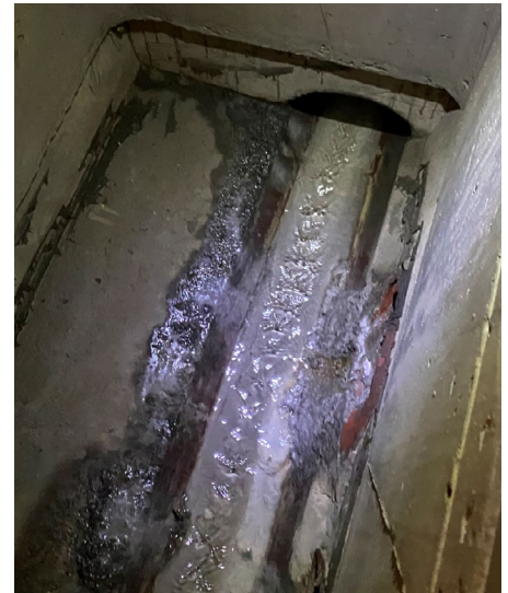
2 months after water jetting
