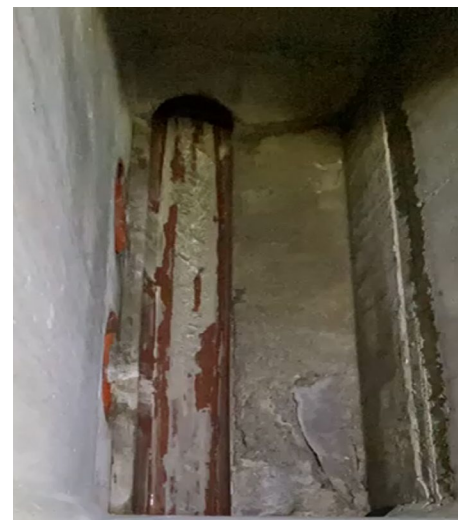
3 months after DrainBot installation
